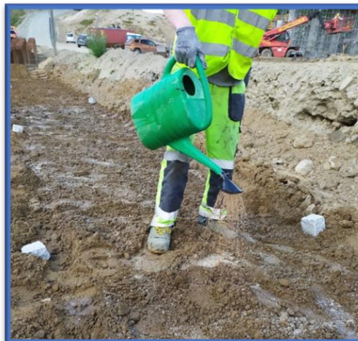
Fig. 1. Manual application of liquid soil stabilisers (emulsion based on plastic waste pyrolysis products – waxes).
